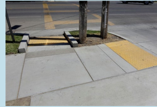
Washington Elementary crosswalk with misaligned ramp
