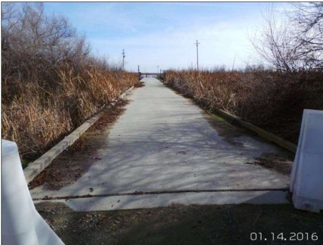
Figure 3-4. Photos of Beaver Damage to Bridge Piles
