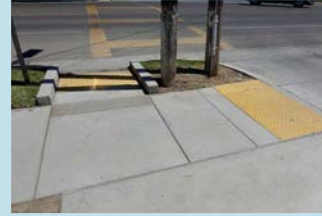
Washington Elementary crosswalk with misaligned ramp
