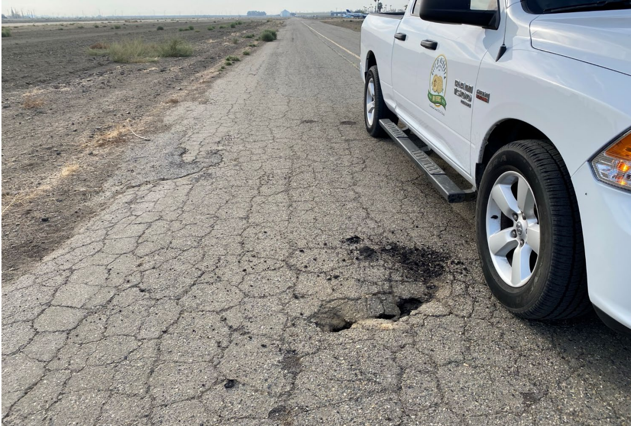
Photograph 4 - Example of collapsed Taxiway pavement.
