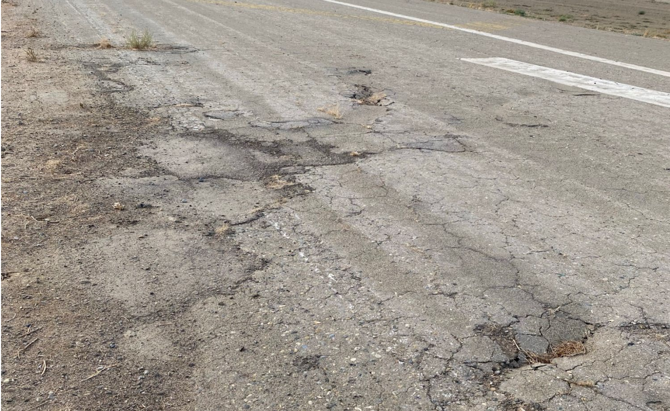
Photograph 2 - Example of the current collapsed Runway pavement condition.
