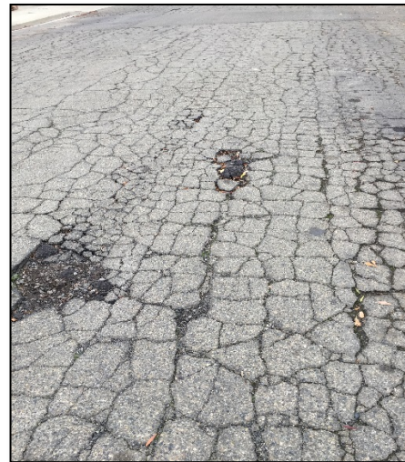
PCI = 12 (Very Poor)
